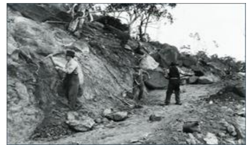
Cutting access track to Jindabyne Dam site, 1950 (Snowy Hydro's online photo library)
